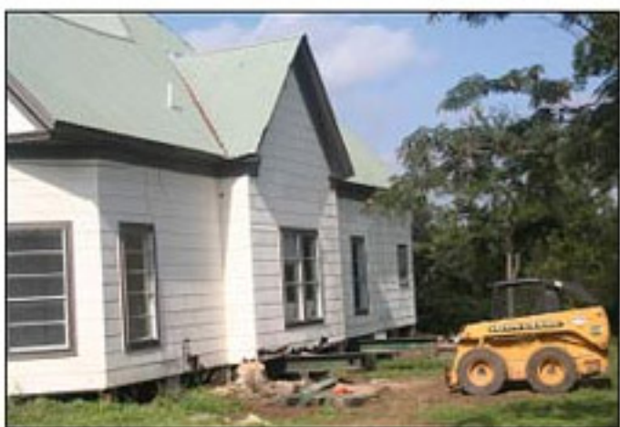
Sturdy metal beams are placed under the 110-year home at 302 Ave. N to move it up the street about 100 feet. A day care will be built on the site where the home, described as the fifth oldest in Marble Falls, once sat.
